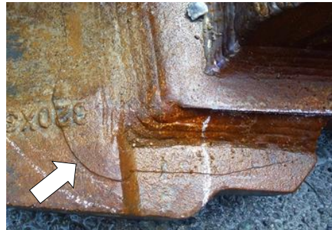
Example of stress cracking.
