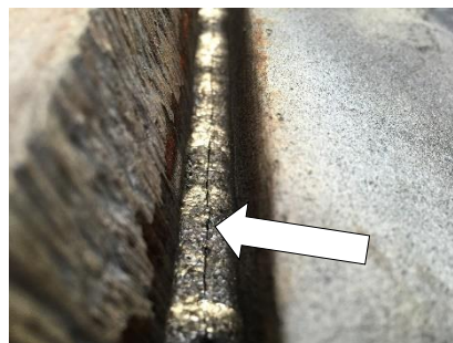
Example of longitudinal cracking.
