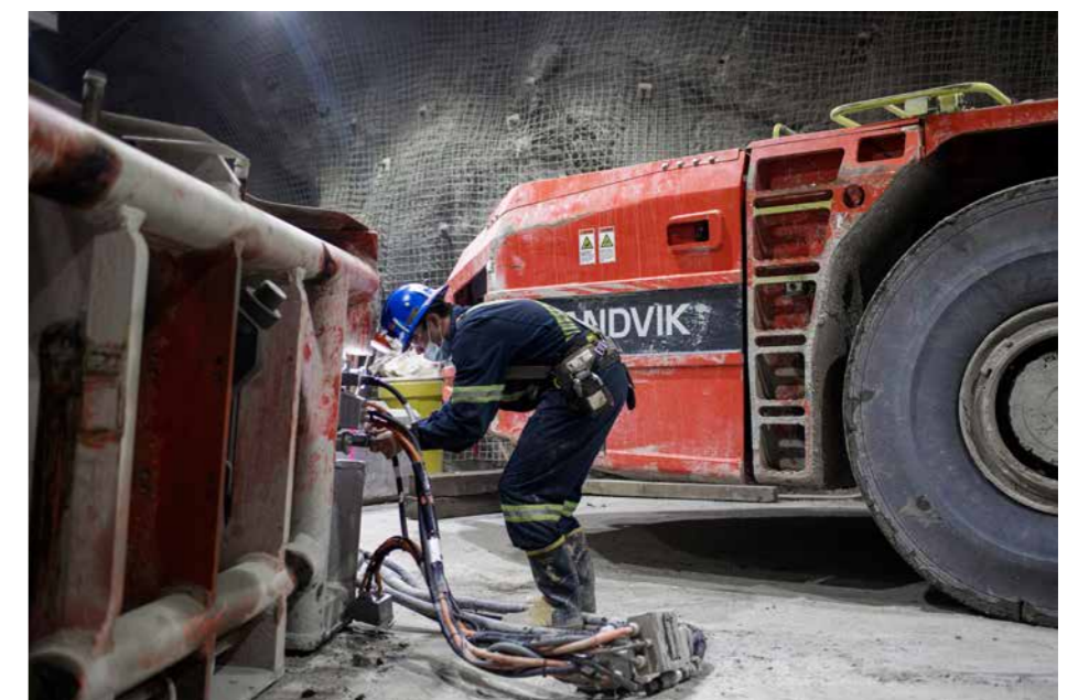
Battery swapping enables New Afton to spread the charging load over longer periods of time, helping to mitigate the aggressive power draw that quick charge solutions have.
